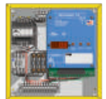
Drive Control Panels
