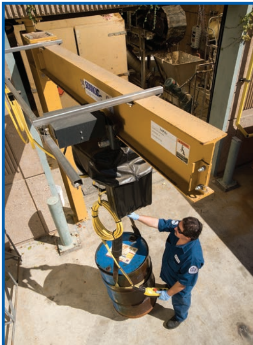
A water treatment plant uses this Spanco Two-Ton 200-Series Full-Cantilever Mast-Style Jib Crane at its receiving dock.
