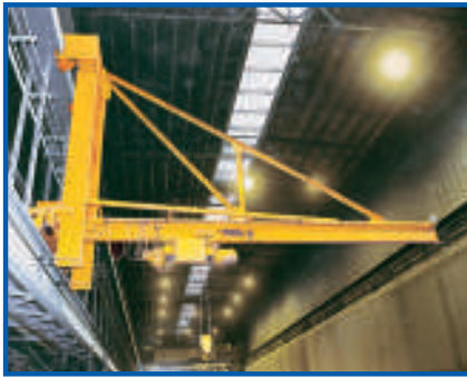
A Spanco 5-Ton Wall-Traveling Jib Crane is installed beneath an existing overhead bridge crane and covers the entire length of the facility.
